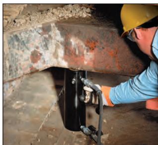
◀ An RAR-506 was easy to position under a bulldozer for repair of frame member.
